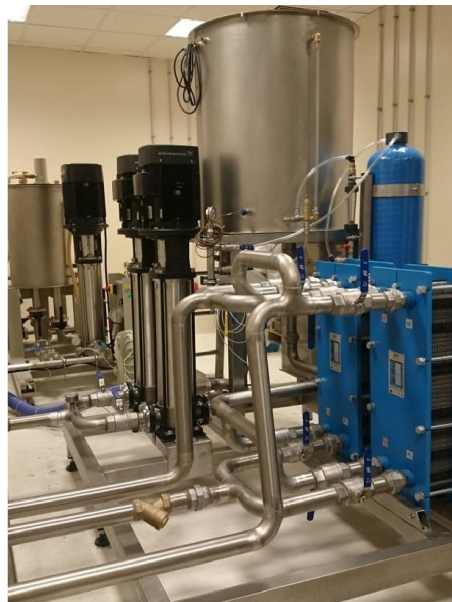
Figure 6. Cooling System of METU-DBL in the Cooling room of TAEA PAF. The cooling water of METU-DBL comes from the main chiller of TAEA PAF. The cooling system of METU-DBL includes two heat exchangers, two pumps, a water tank and a resin tube.
